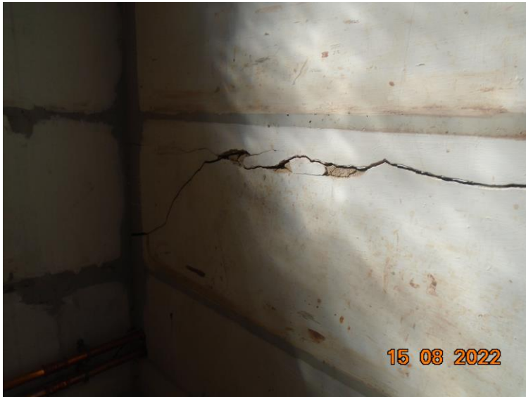
Structural cracking to partition wall between art room stores.
