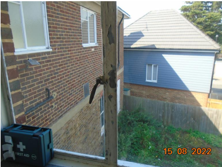
Deteriorated paint to steel crittall windows.
