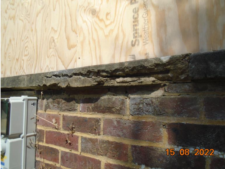
Cracked and spalled concrete subsill below recreation room 3 window.
