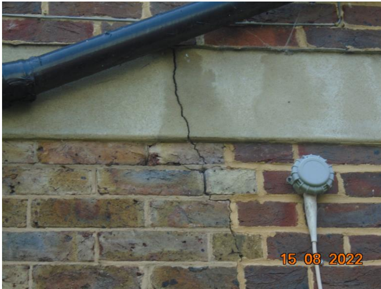
Cracking to rear concrete band and masonry.
