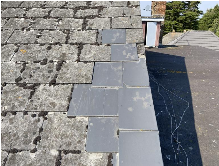
Broken asbestos fibre cement slates, and replacement slates to rear east verge.
