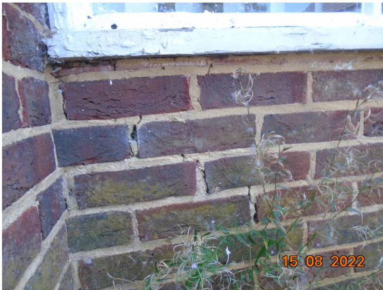
Stepped cracking to rear wall of recreation room 3.
