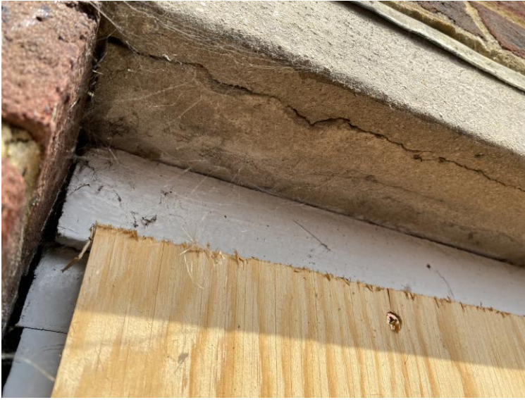
Cracked concrete lintel above recreation room 3 front window.
