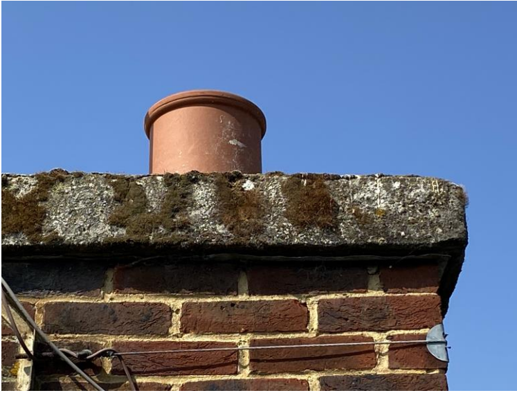
Cracked concrete coping to northwest chimney stack.
