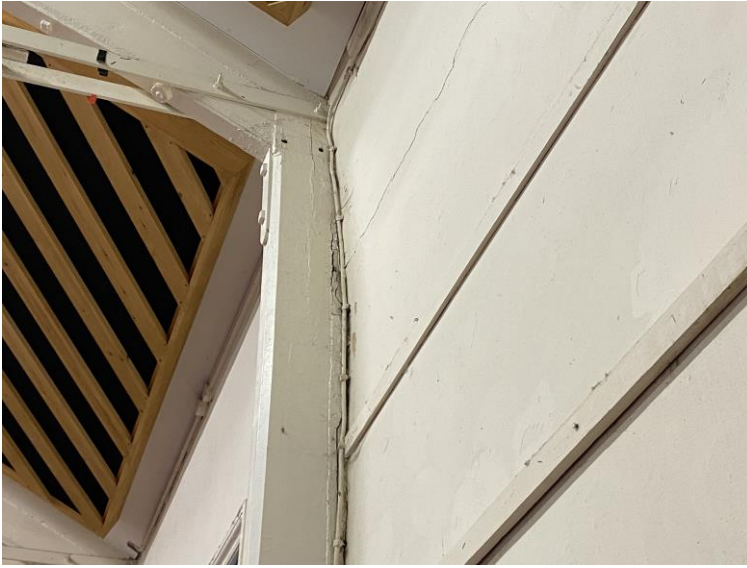
Bulging to west wall of gym.
