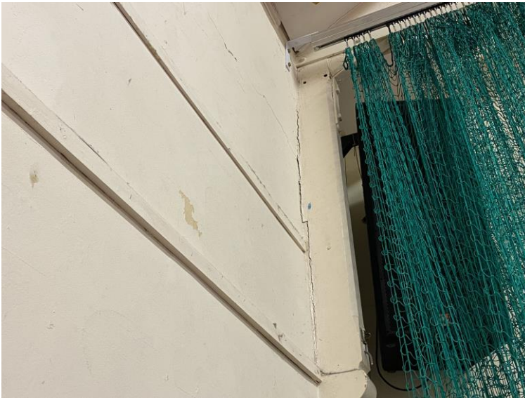
Bulging to west wall of gym.
