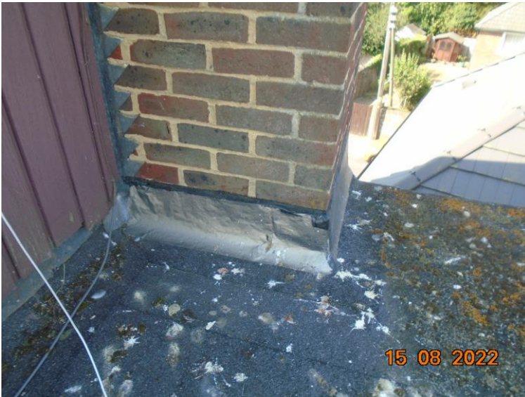
Low quality flashband to northwest chimney stack.
