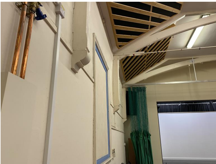
Bulging to west wall of gym.
