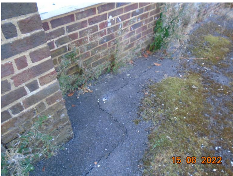
Sunken tarmacadam to rear.
