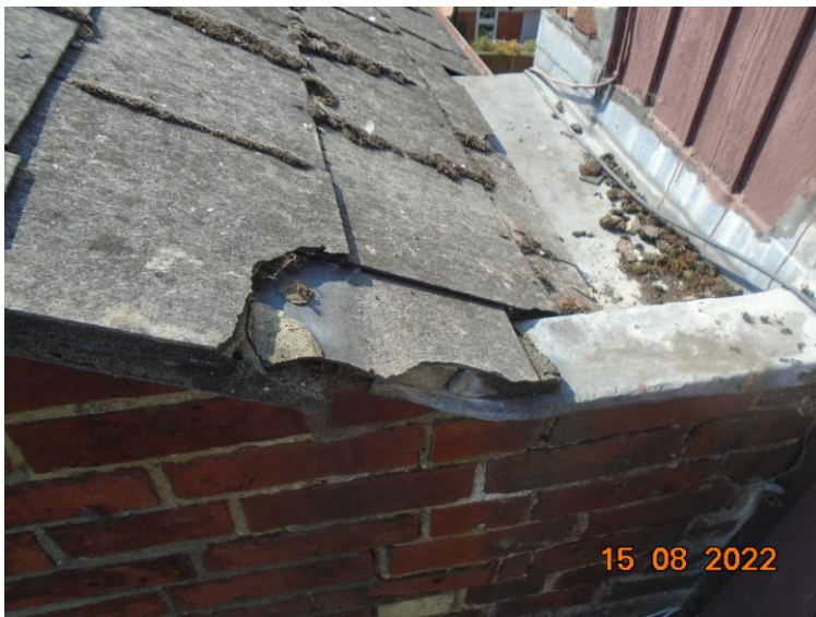
Broken slates to rear west verge.
