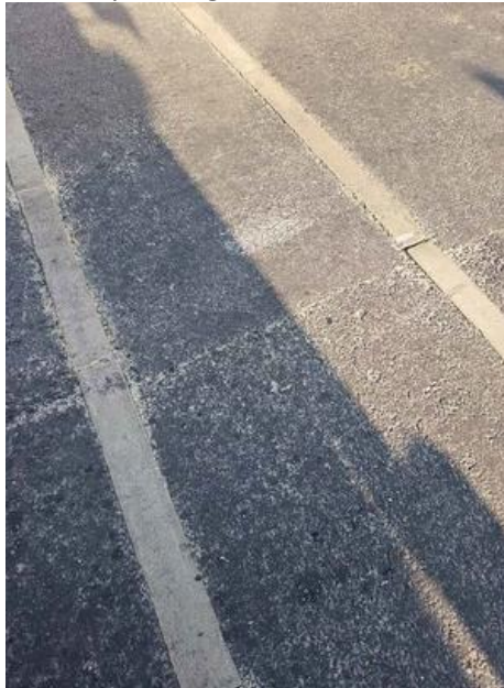
Evidence of ground out on ramp
