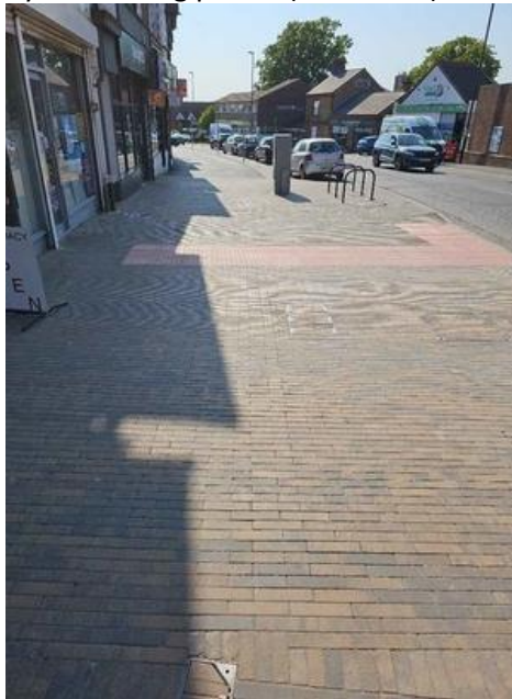
No drainage in this location. Wet weather visit required.
