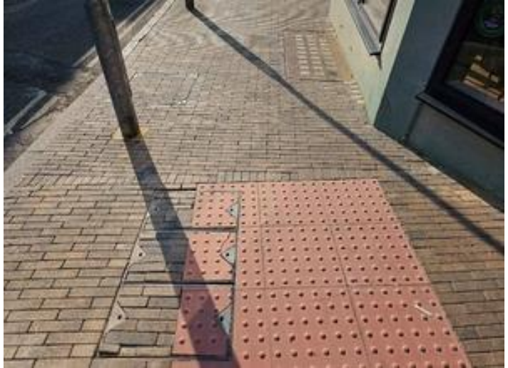
A row of stretcher course would have been better
