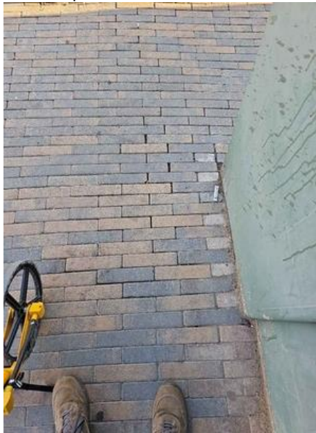
Poor finish on blocks. Open joints.
